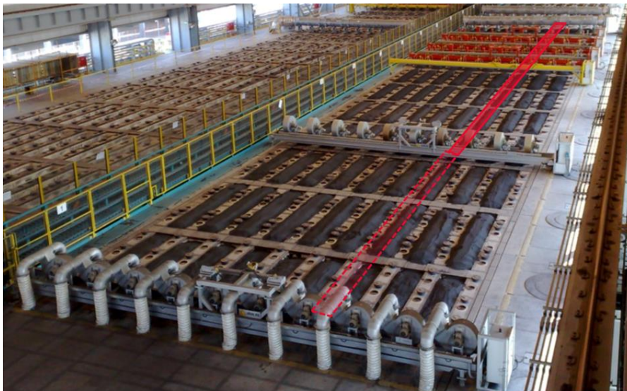
Figure 1. General view of an open Anode Baking Furnace and representation of the fire geometry used in the model.
